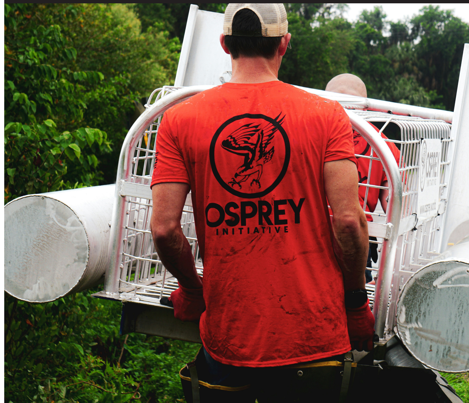
Installing a trash guard to reduce marine debris, in Ellenton, FL. with the Tampa Bay Estuary Program.
