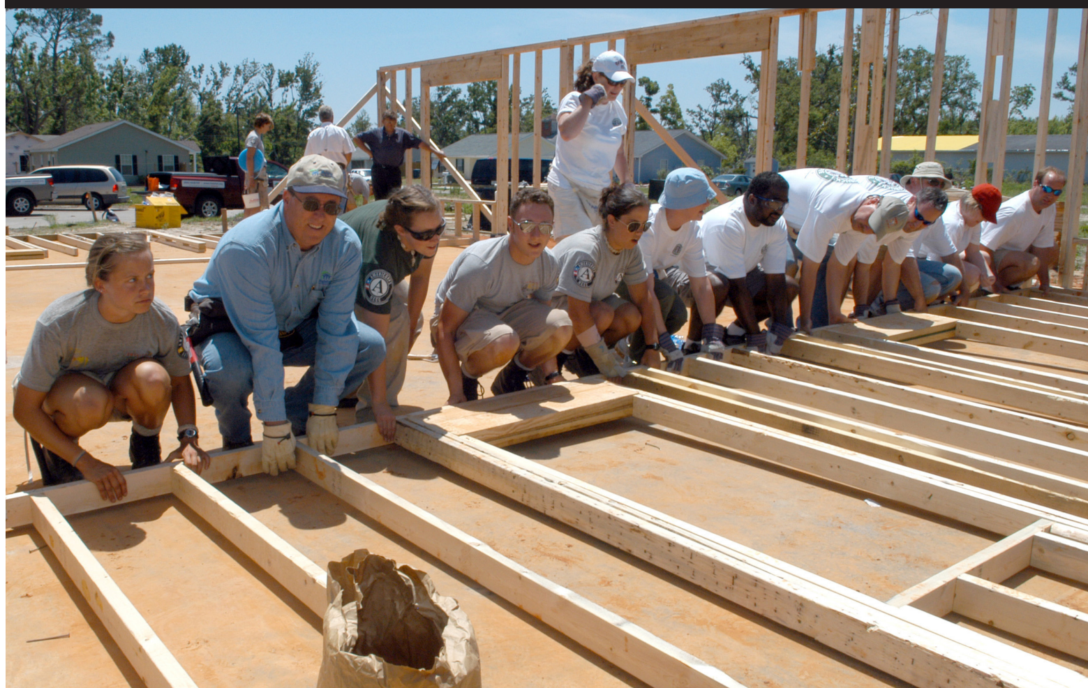
Habitat for Humanity, AmeriCorps NCC and Starbucks corporate volunteers build a bunkhouse for volunteers assisting in recovery efforts, Gulfport, Mississippi, 2006. Photo courtesy of George Armstrong/FEMA
