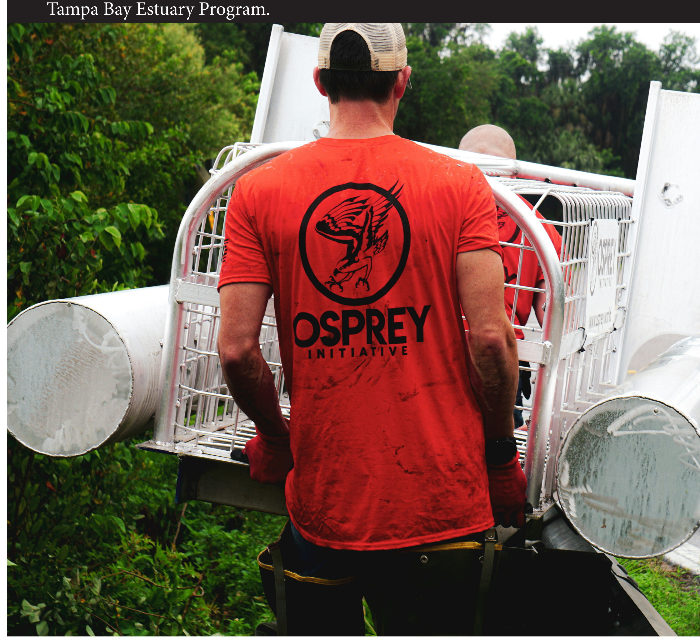
Installing a trash guard to reduce marine debris, in Ellenton, FL. with the Tampa Bay Estuary Program.
