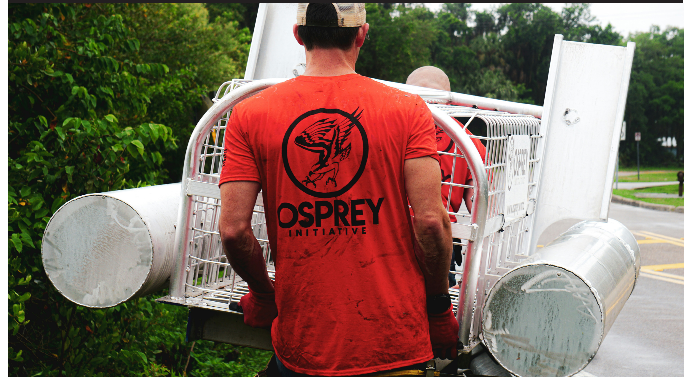
Installing a trash guard to reduce marine debris, in Ellenton, FL. with the Tampa Bay Estuary Program.
